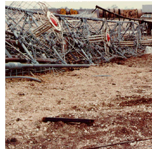
Final antenna (“basket”) section of Missouri City antenna (section that dropped).
